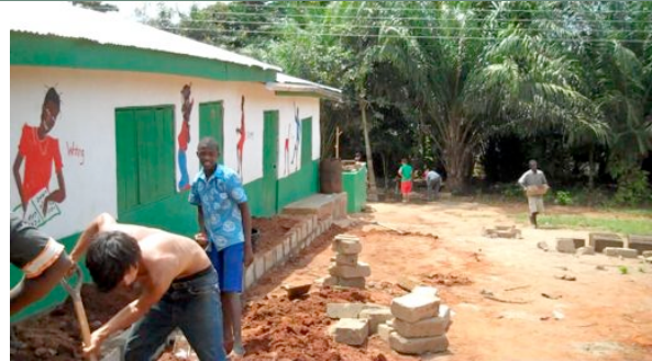
Working on the second 2-classroom block, and our farming site is behind those trees!
